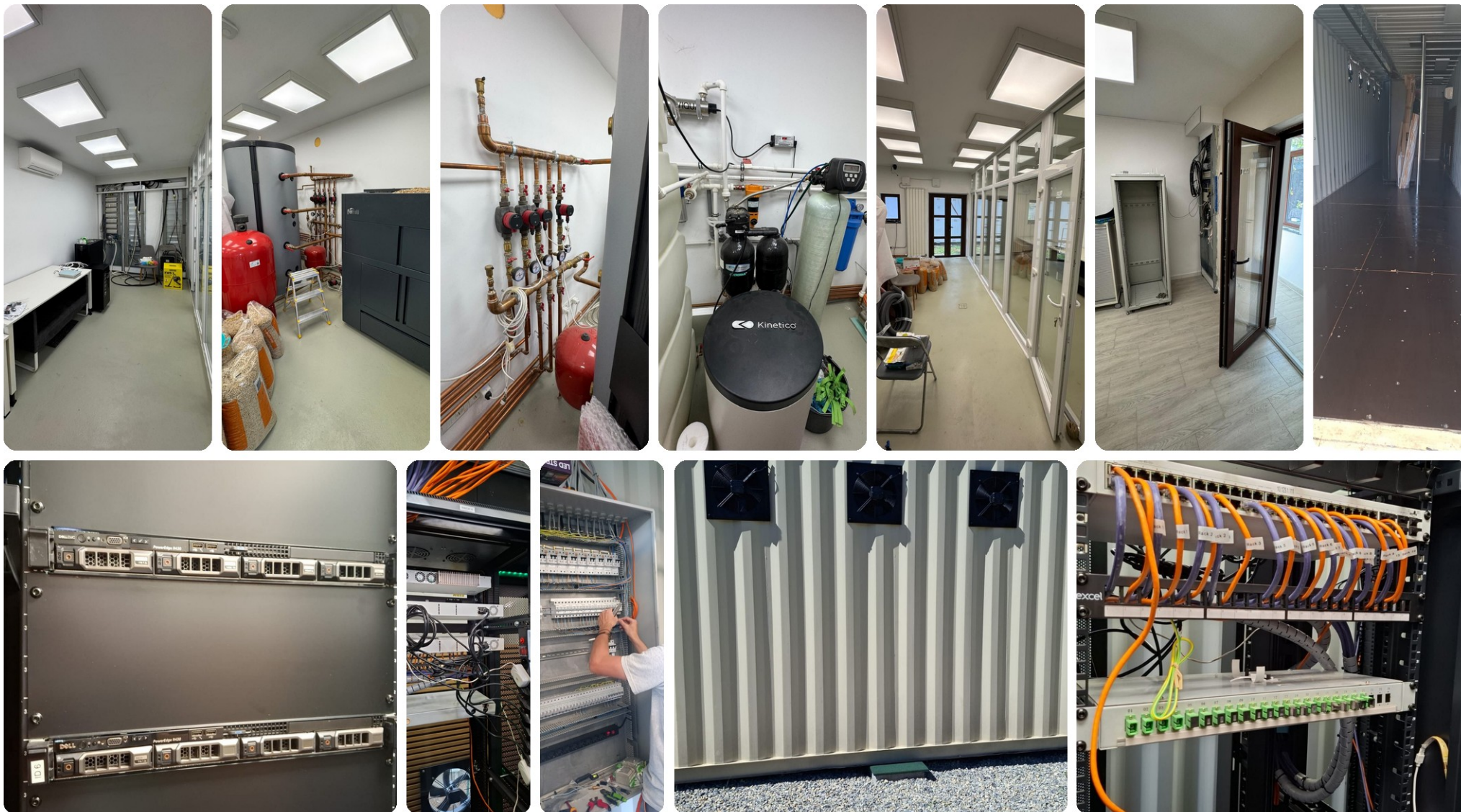
Technical building on site: ion-exchange water softening, heating and hydraulics, glazed office partitions; the container fitted out with cabinets, patch panels, power distribution and cooling.
