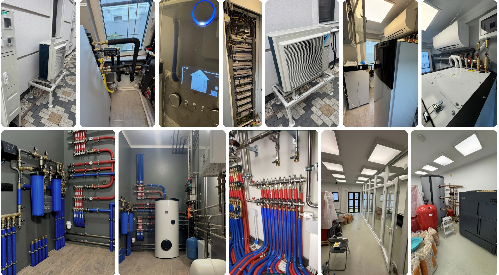
Outdoor heat pump units on brackets, floor-standing indoor units, underfloor manifolds in red and blue, hot water cylinders, distribution boards, KNX actuators and the smart thermostats on the wall.
